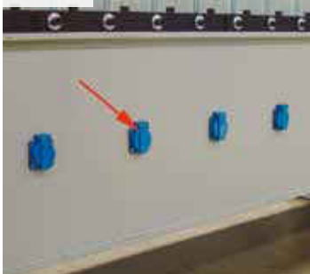
4 Additional sockets for heaters.
