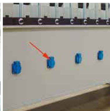
4 Additional sockets for heaters.
