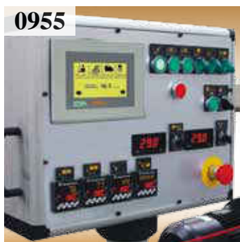
0955 Centralised electronic speed control of several machines.
