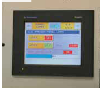
IR lamps power regulation from the control board.
