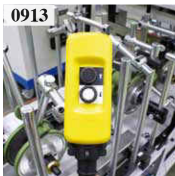
0913 Auxiliary cable command for the control of the conveyor to facilitate the wrapping tool adjustment operations.
