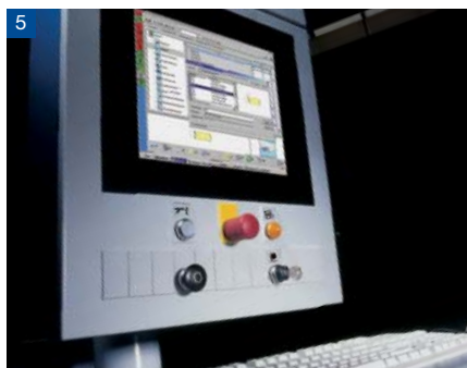
200 series: contactor control 500/600 series: powerControl In accordance with IEC 61131/3 optionally: Siemens S7
