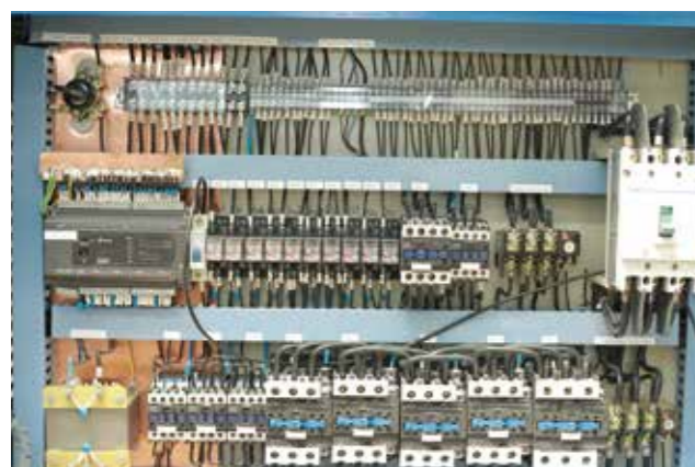
Main electronic components use schneider
