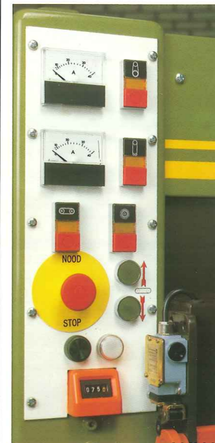
Control panel electricity
