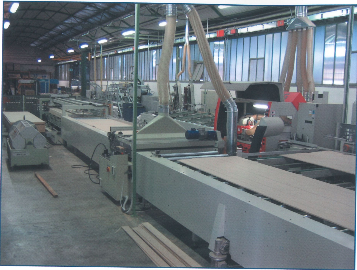
15 - Multiblade saw panel loading and unloading.
