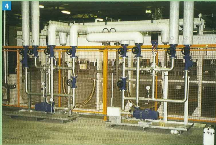
4 Sekundärstationen zur Temperaturregelung. Secondary unit for temperature regulation.
