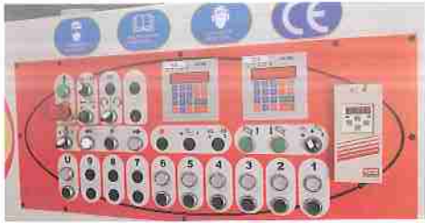
▲ Control panel German made Moeller electrics. A Germany Moeller brand switch giving you reliable and distinct control.
