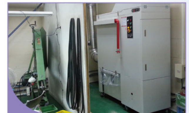
LS-500A In The Metal Sheet Processing Factory
