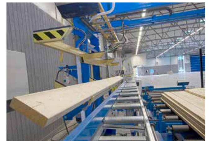
Board is ready to be slid or flipped down to the infeed bench.
