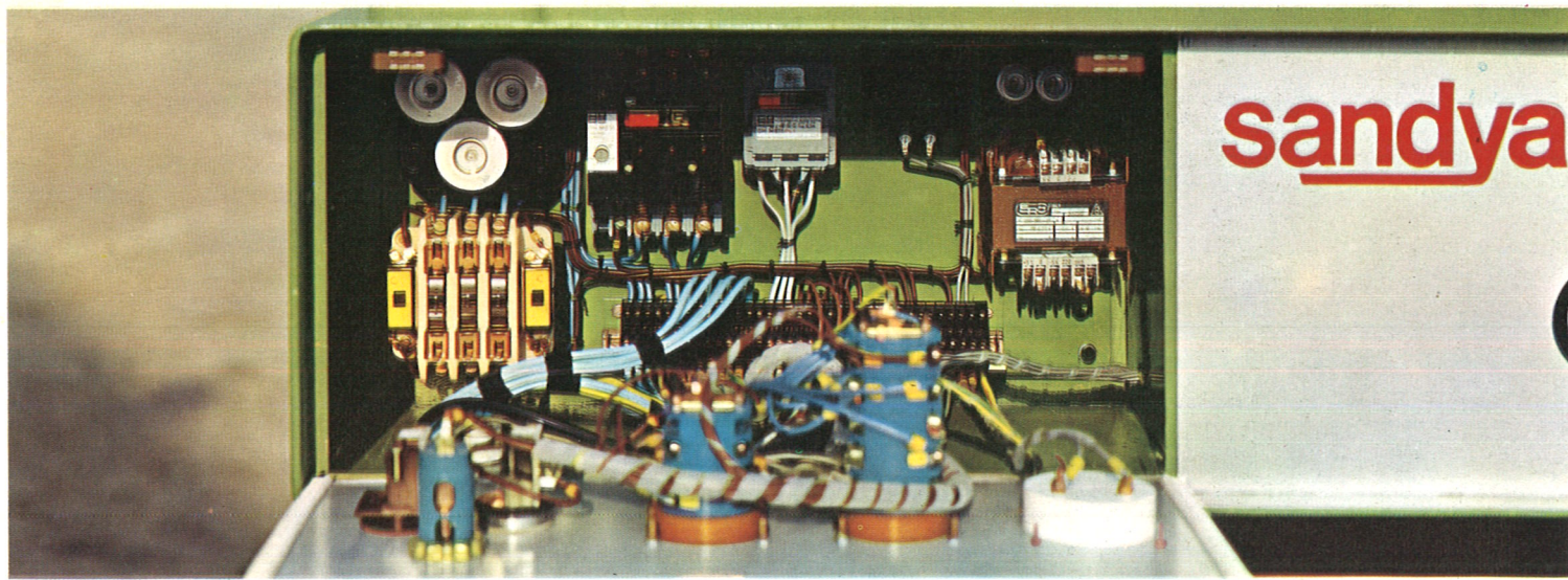
Electric installation on a panel in sealed box: note the motor protection equipment.
