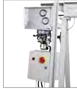
Detail of the control panel.
