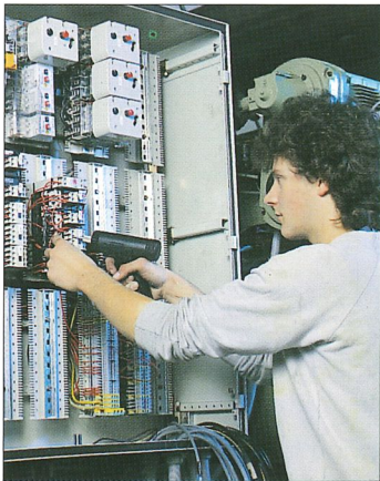
The electrical cabinet, the control center of the Profimat.
