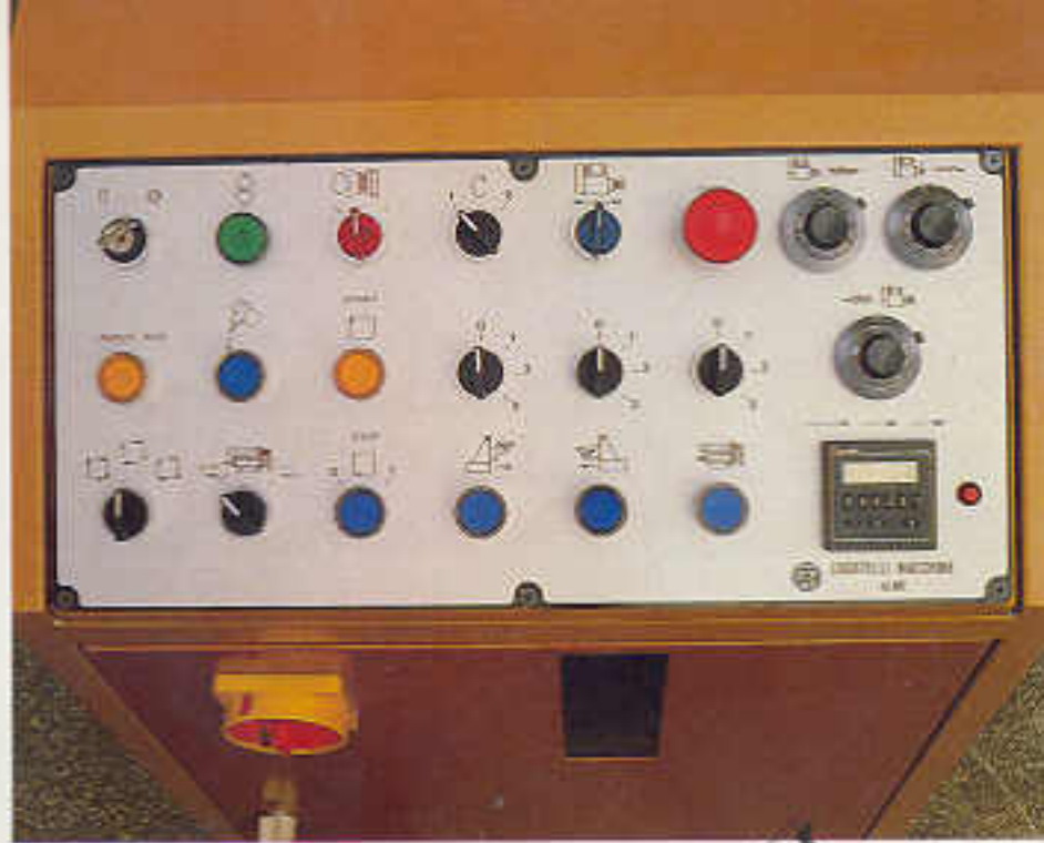
Programmed logic control panel
