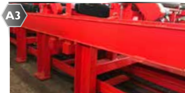
Elevated rails with automatic system for waste cleaning.
