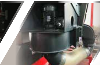
Additional sawdust exhauster system with ventilator on machine.
