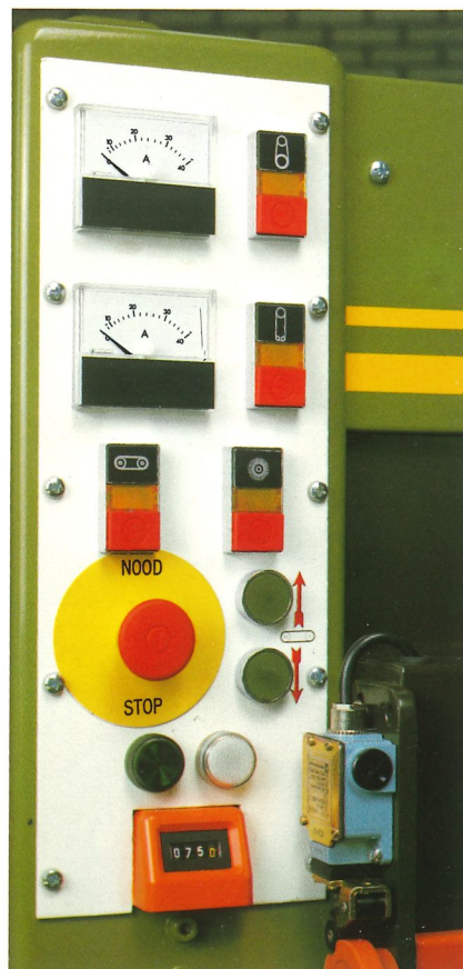
Control panel electricity
