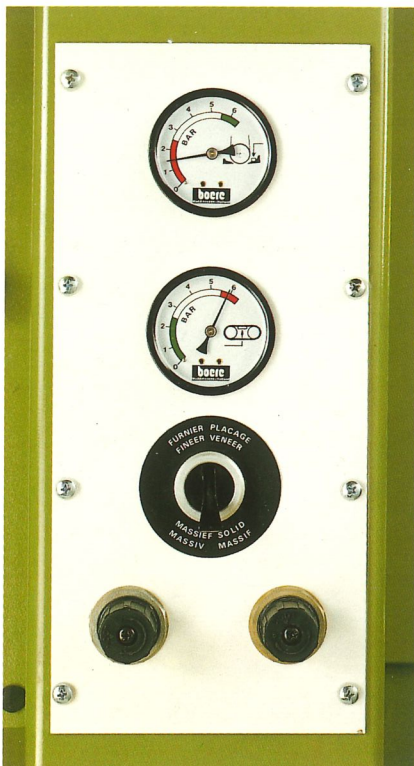
Control panel pneumatics
