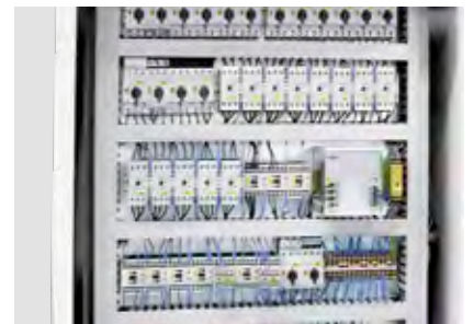
Freestanding switch cabinet with cooling unit and separate frequency converter per motor
