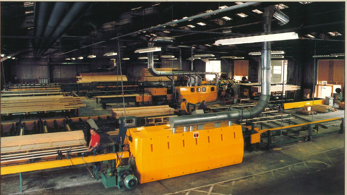
A turnkey high production mechanised moulding line installed at Montague L.Meyer (London) Ltd., Barking, Essex.
