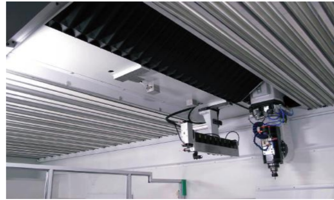
Bellow-type roof for dust containment
