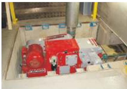
RHZ 400 S set up below ground
