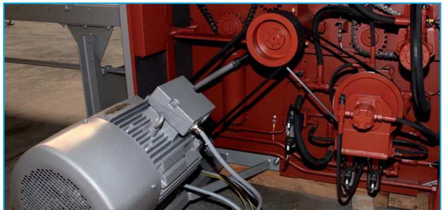
Fig. 11: Drive motors up to 75 kW driving the saw shaft via V-belts
