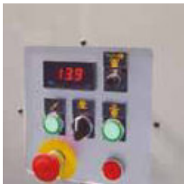
Speed regulation through INVERTER with digital display.
