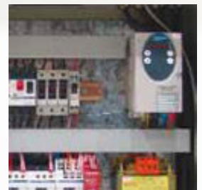
Speed regulation through inverter with digital display.
